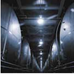
Fill level measurement in tanks
